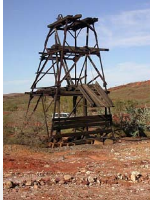
Old head frame of underground workings at Whim Creek Mine, WA (2008, Public Domain)
