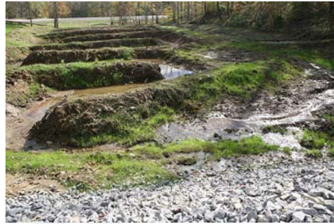
Acid mine drainage in Ohio, USA, is treated through limestone dams and channels that neutralise pH (Wayne National Forest 2010, Wikimedia Creative Commons)
